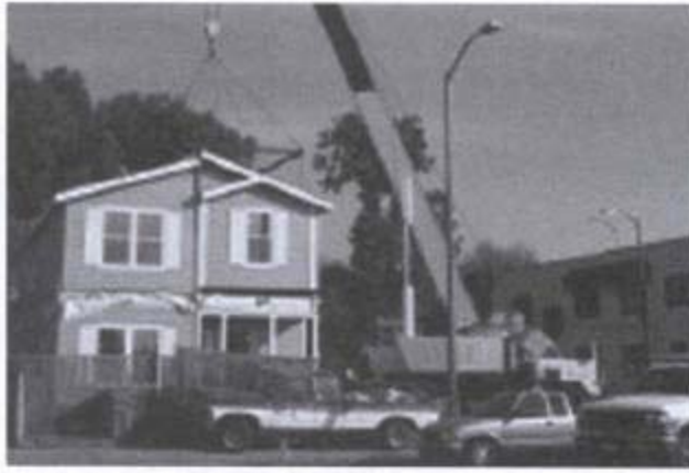
Installation of the first and second floor modules is normally completed in one day.
